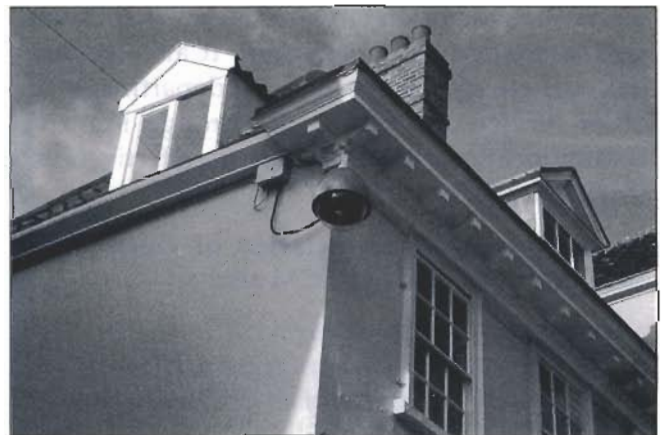
CCTV on an historic building
